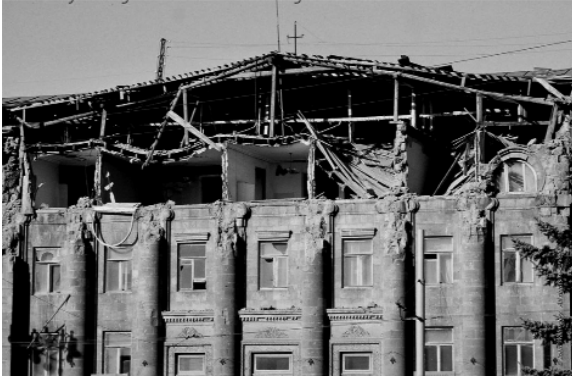
The building of Leninakan City Council of the Kommunist Party of Armenia after the Earthquake of 1988. It was built in 1952-1953. Architect: Zaven Bakhshinyan (1908-1989)
